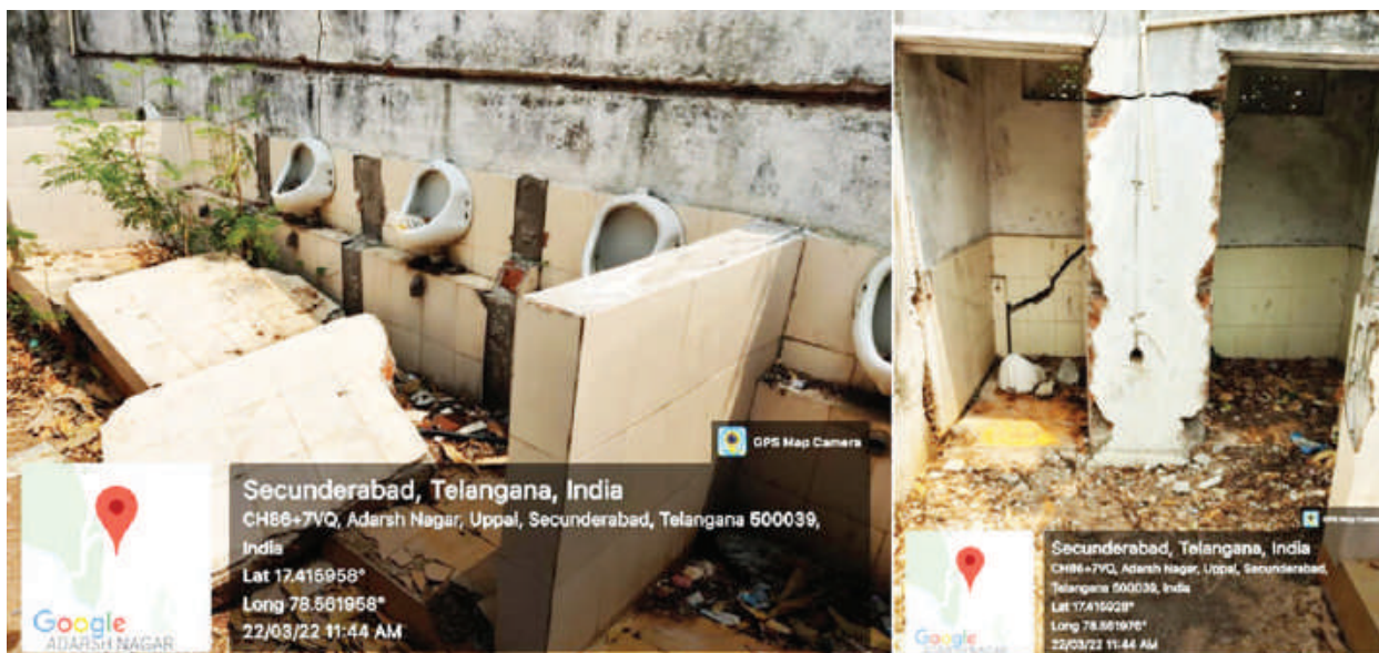
BEL renovated school toilets became dysfunctional due to lack of operations and maintenance by school authorities of Chilkanagar
