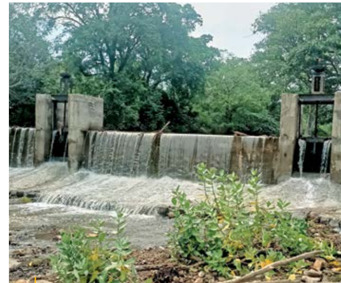
Water retention in check dams constructed on natural streams in MM Hills Wildlife Sanctuary, Karnataka.
