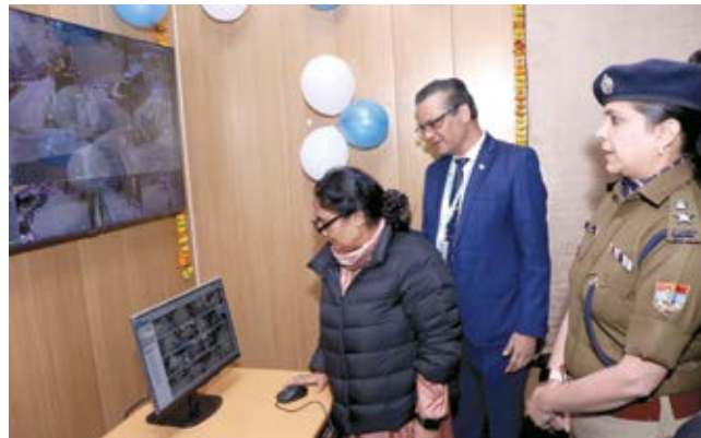
CCTV Surveillance System installed & commissioned by BEL in Kotdwara, Uttarakhand, was handed over to Kotdwara State Police in the presence of Hon'ble Speaker, Uttarakhand Legislative Assembly
